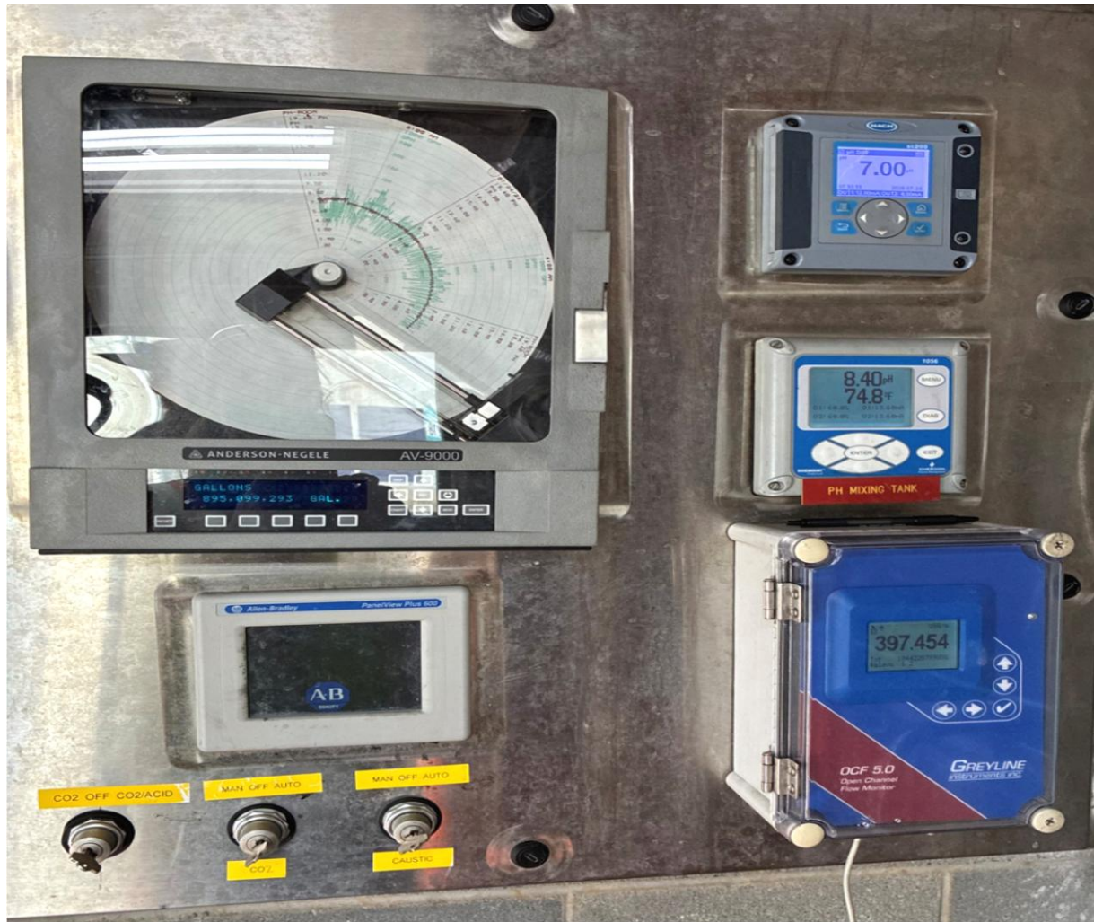
Facility's pH/flow monitors
