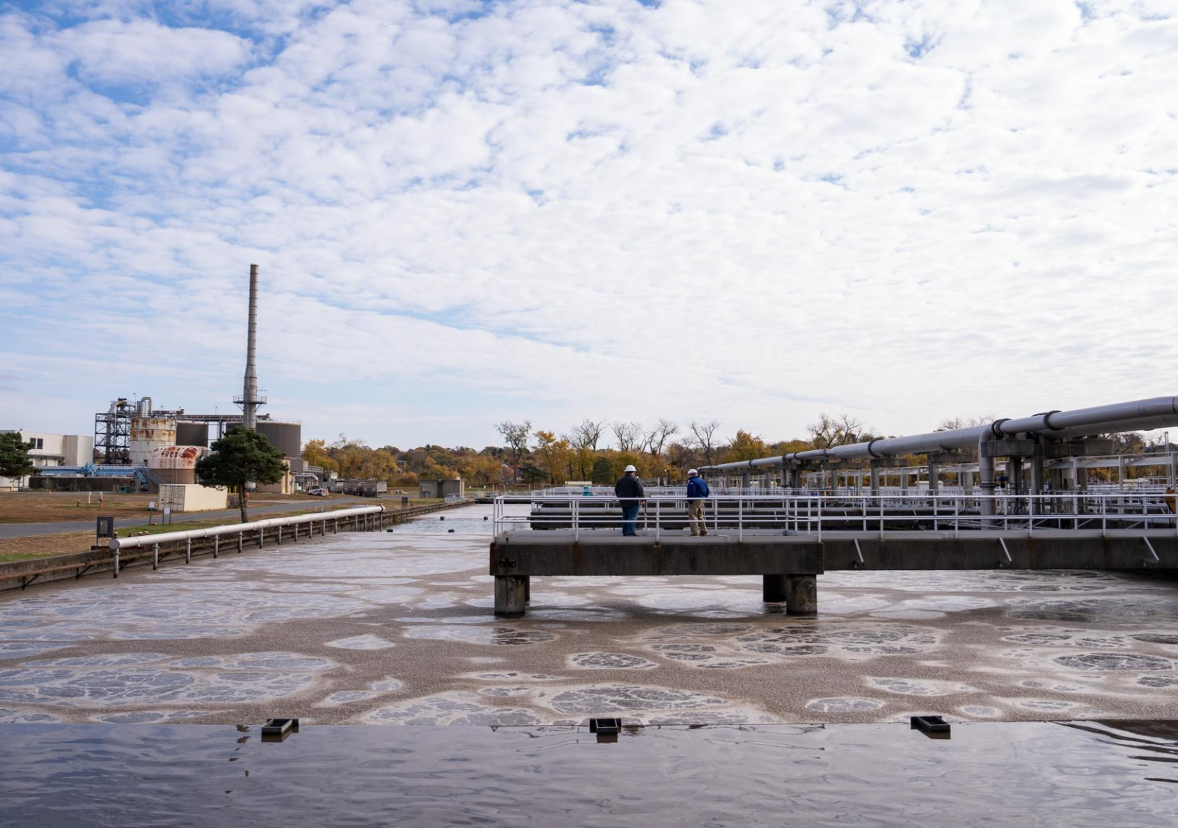
Aeration Basins, Bondi's Island
